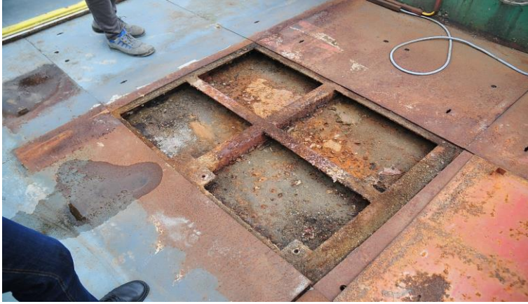
Figure 5: After the superstructure was removed, severe corrosion damage was found under the cargo holds (© Semrad).
