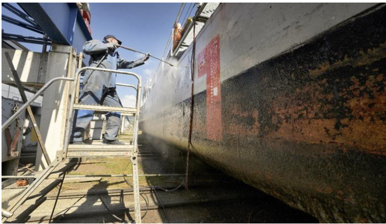
Figure 3: Cleaning the ship's hull from shells and corrosion (© Zinner).
