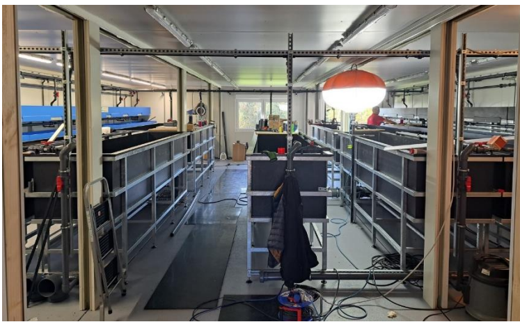
Figure 8: In October, all aquaculture components in the container were prefabricated and the piping was 60% completed (© Kunststoff Spranger GmbH).
